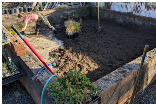
Scraped to the floor
